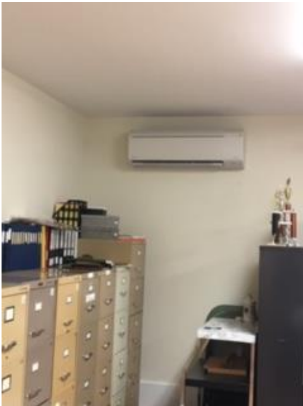
One of three installed heat pumps.
