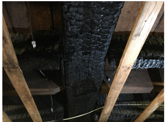
An example of a burnt beam under the old Hampden Academy brick building
